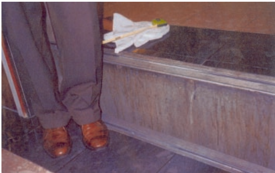
Misleveling problems of an elevator are often not noticeable from the entryway.
